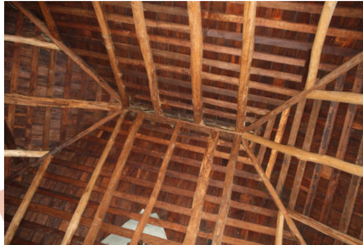
Figure 14: Looking up at the hand sawn timber framing of the main roof.
