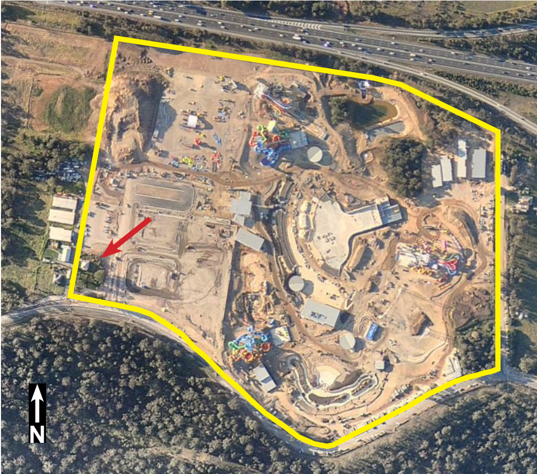
Aerial view showing the location of the Policeman's Cottage (marked by the red arrow) with the Wet n' Wild development site.
