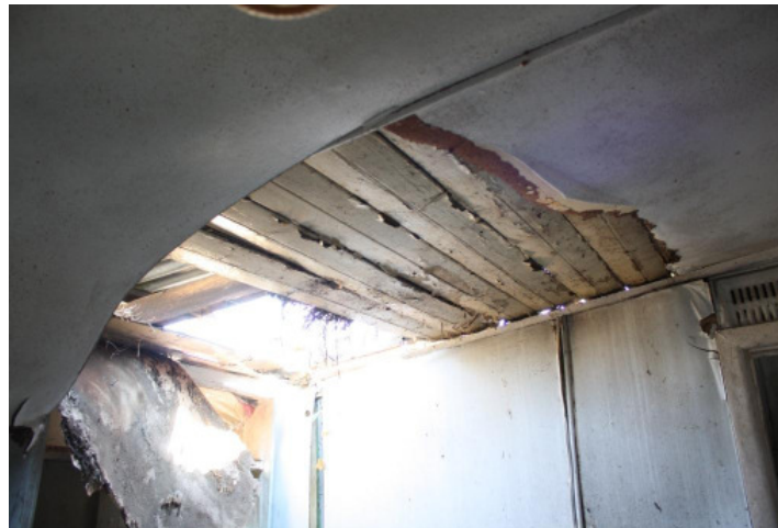
Figure 16: Space 7 - View of the earlier timber lined ceiling below the later ceiling lining.
